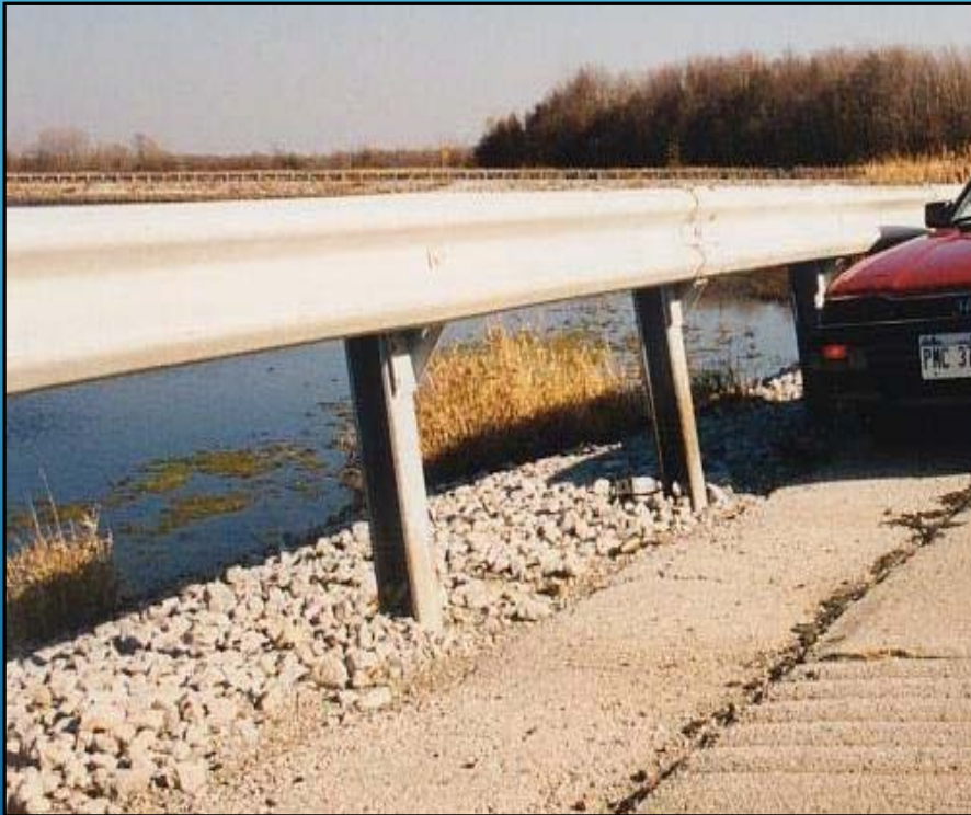
Rail too high
