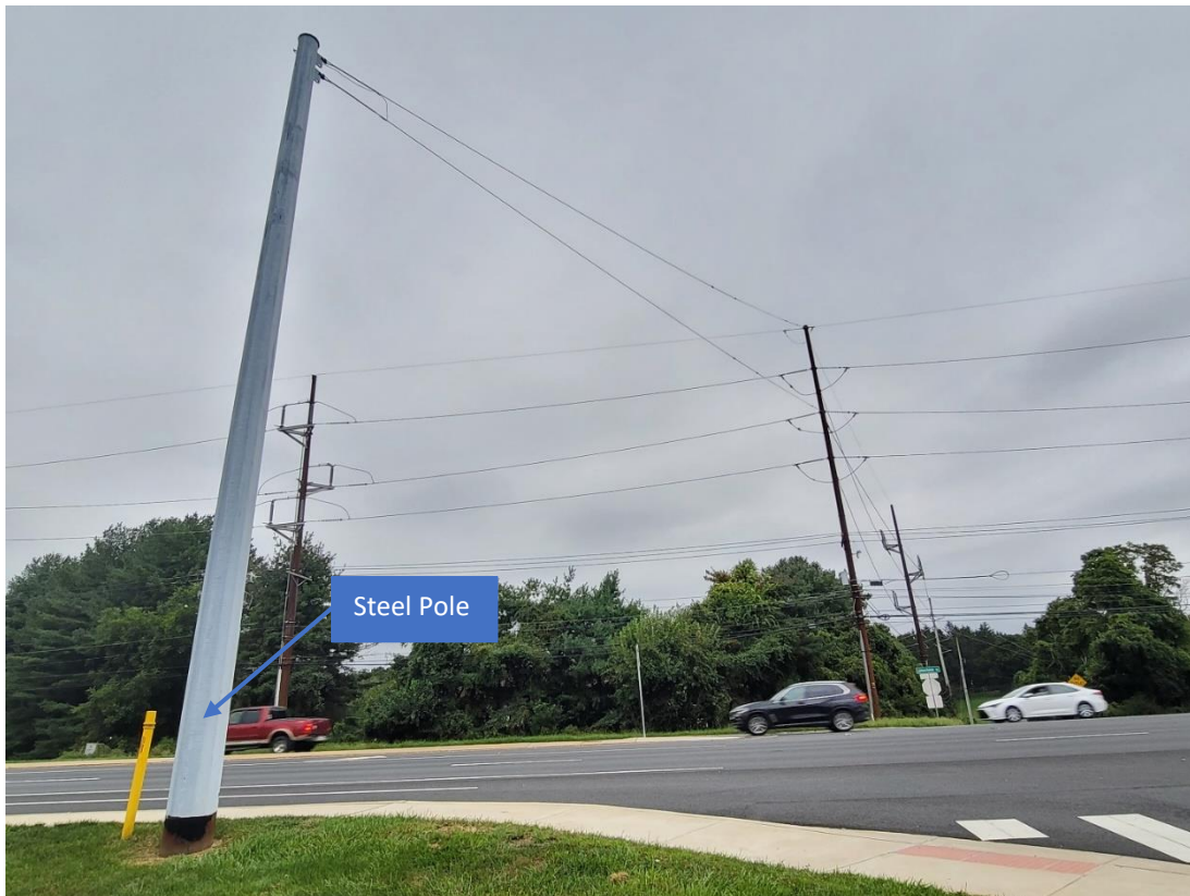
Figure 2-4: Steel Pole (Guy Pole)
