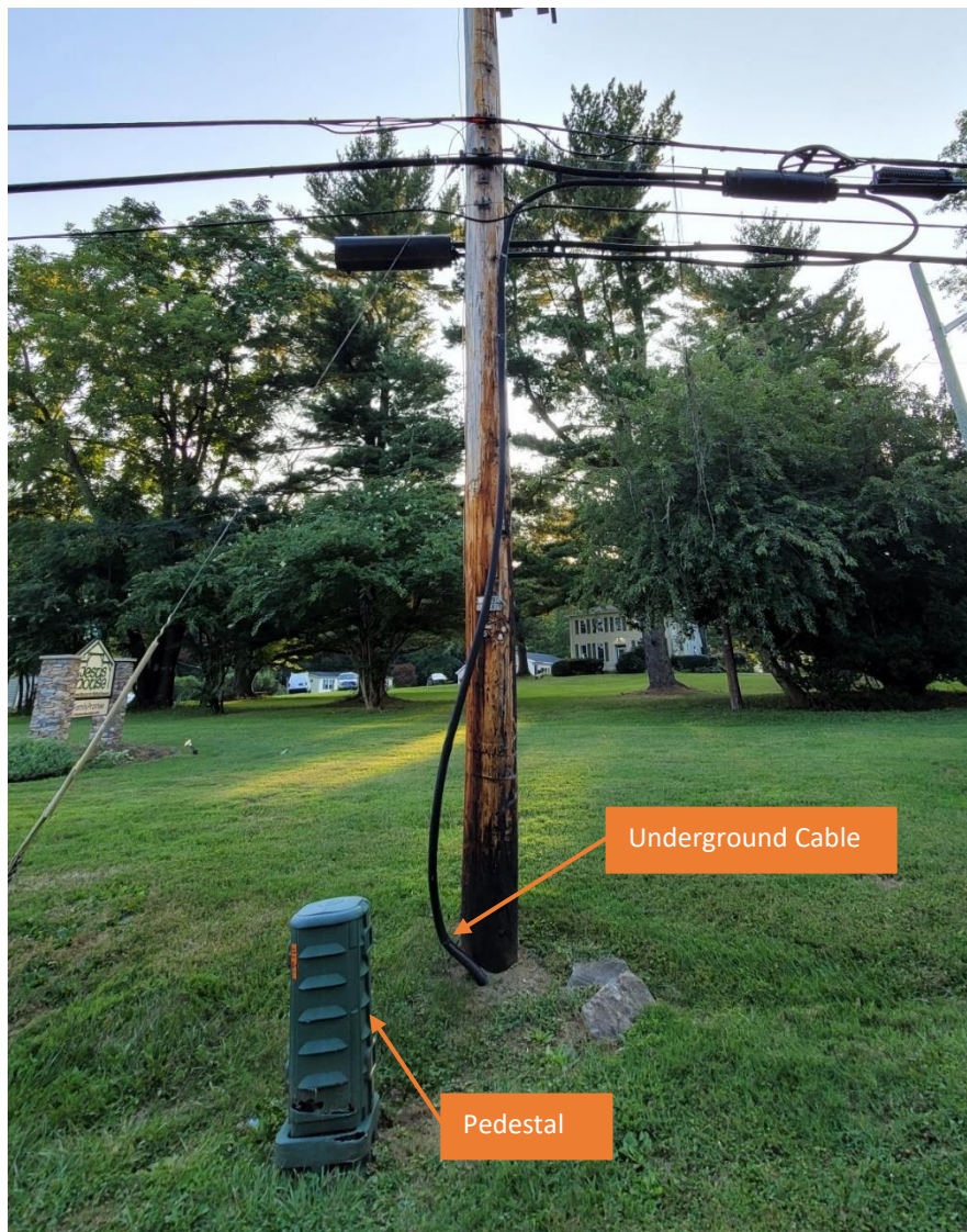
Figure 5-1: Aerial to Underground Cable and Equipment
