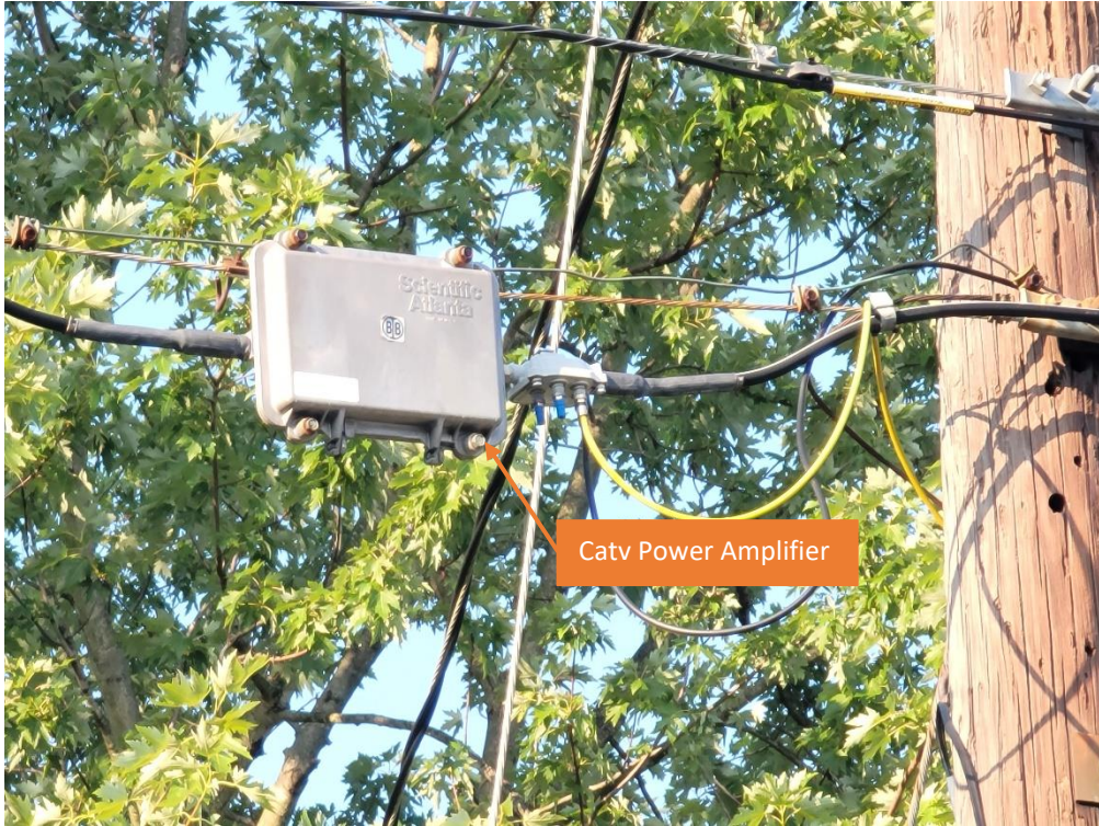
Figure 4-28: CATV Power Amplifier
