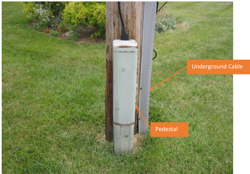
Figure 5-3: Aerial to Underground Cable and Equipment
