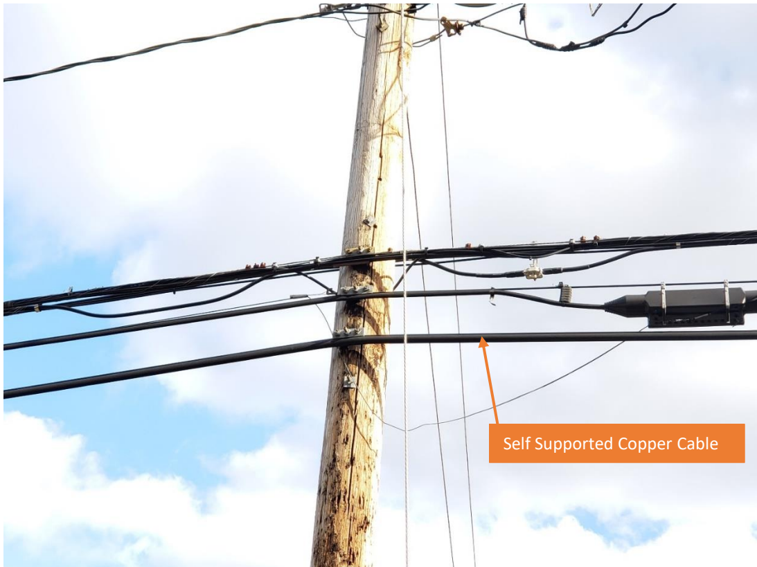
Figure 3-2: Self Supported Copper Cables
