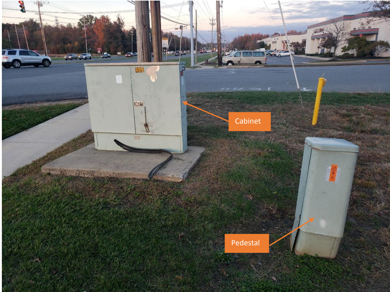
Figure 5-4: Aerial to Underground Cable and Equipment
