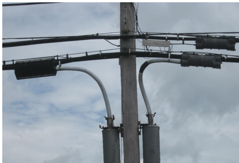
Figure 2-11: Verizon Cables and Equipment
