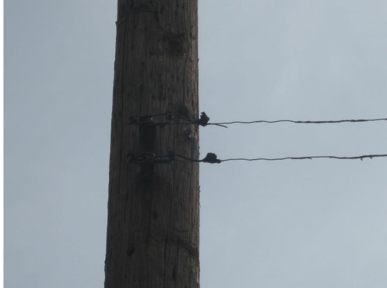
Figure 3-12: Retired Fire Department Cables
