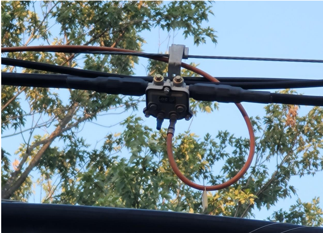
Figure 4-29: CATV Drop Box/Terminal
