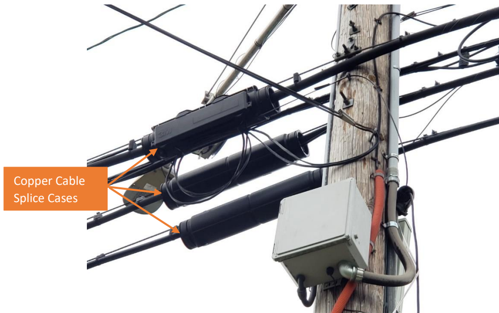
Figure 4-5: Copper Cable Splice Cases
