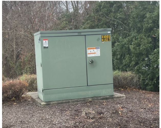
Figure 5-1: Ground mounted transformer with door and Delmarva Power identification number.
