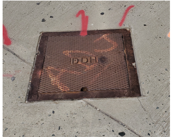
Figure 10-2: DeIDOT junction well lid (DDH denotes Delaware Department of Highways).
