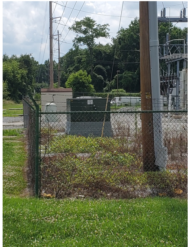
Figure 11-2: Substation perimeter fence.
