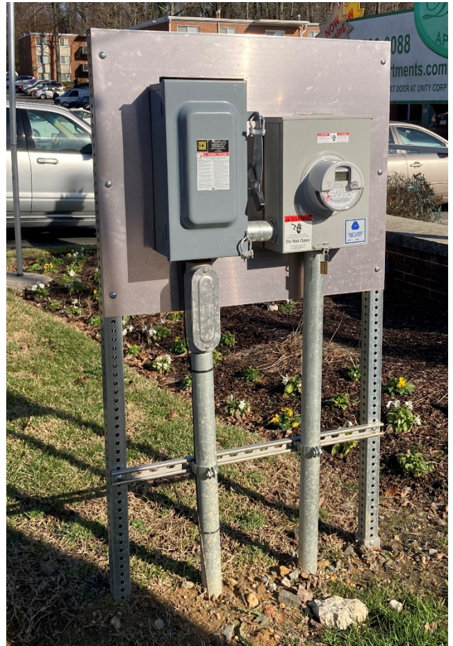
Figure 7-1: Electric service meter on pedestal for DeIDOT facility.
