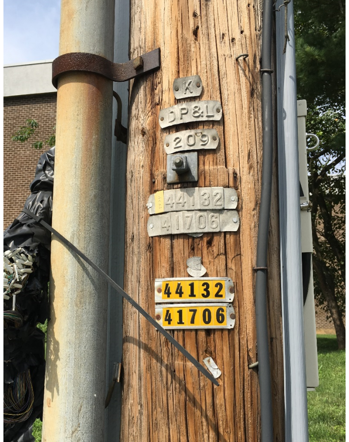
Figure 8-1: Utility pole with various conduit drops for electric and communication facilities.
