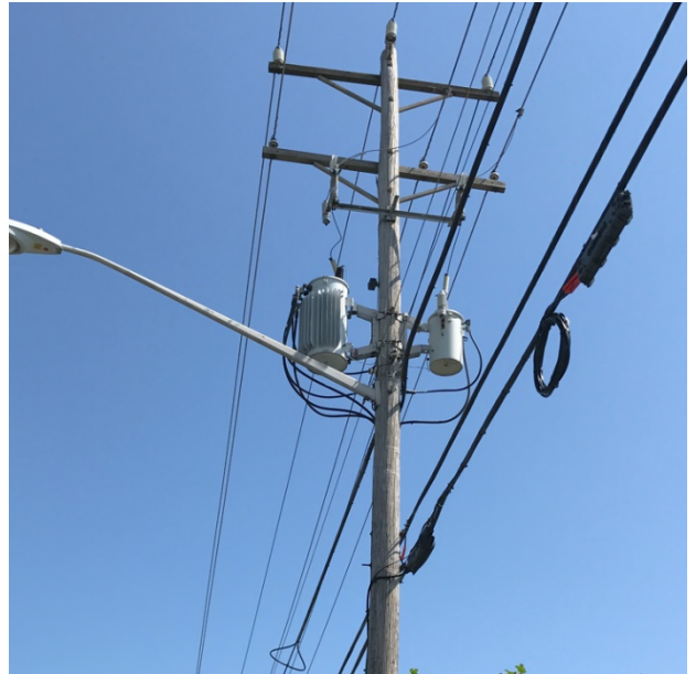
Figure 4-1: Two aerial transformers on utility pole. Service being provided to pole-mounted streetlight.
