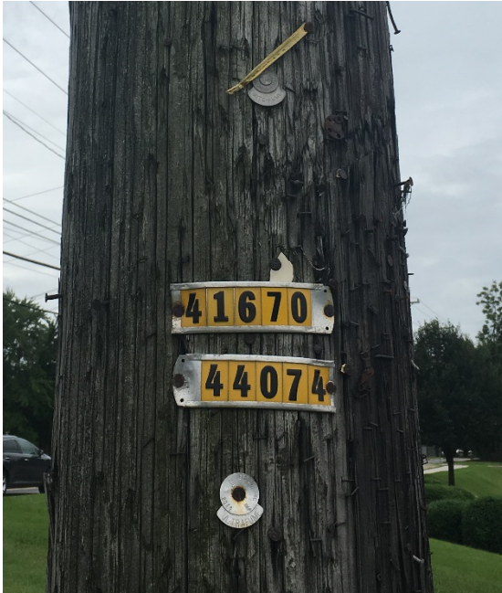
Figure 6-1: Utility Pole with Delmarva Power pole number
