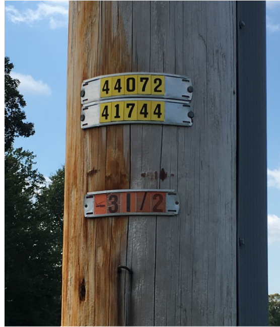
Figure 6-2: Utility pole with Delmarva Power pole number (top) and Verizon pole number (bottom)
