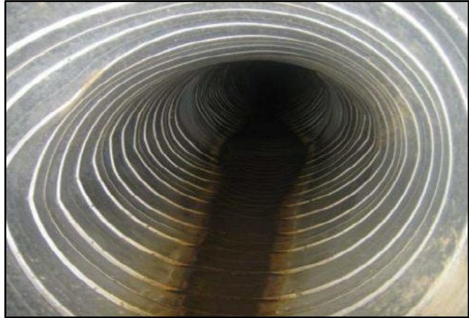
Deflected Pipe. Image Courtesy of Simpson, Gupertz & Hager
