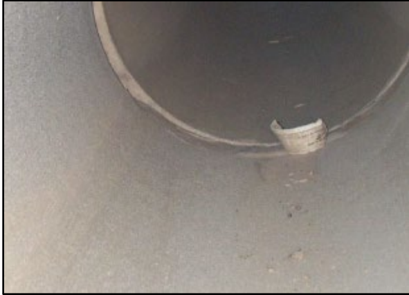
Concrete Joint Separation. Image Courtesy of Simpson, Gupertz and Hager
