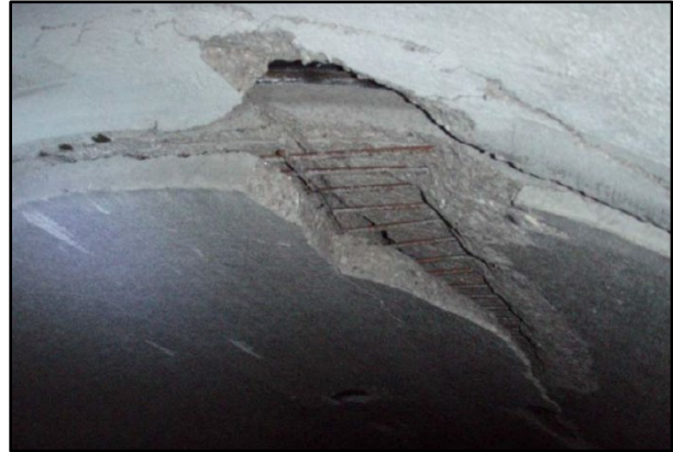
Slabbing. Image Courtesy of Kentucky Transportation Center
