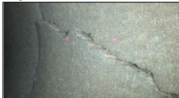
Crack with Vertical Offset. Image Courtesy of Kentucky Transportation Center
