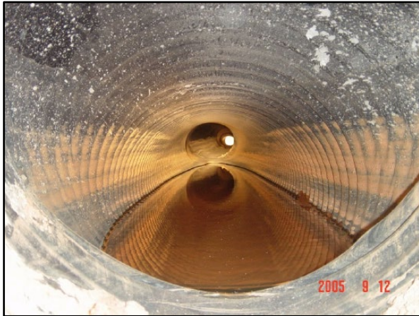
Misalignment. Image Courtesy of California Department of Transportation
