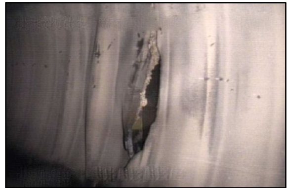
Hole in Pipe. Image Courtesy of Kentucky Transportation Center
