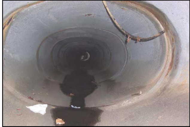
Large Concrete Joint Separation.
