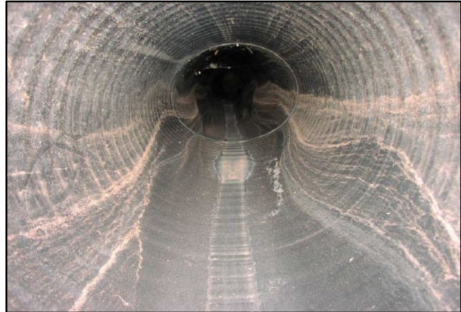
Pipe with Over 10% Deflection. Image Courtesy of Simpson, Gupertz & Hager
