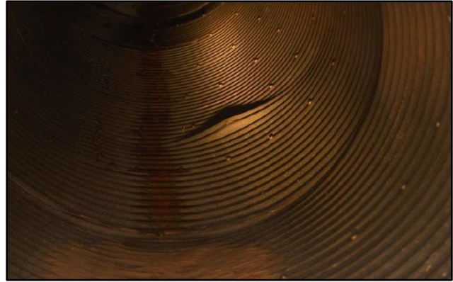
Dent in Pipe. Image Courtesy of Simpson, Gupertz & Hager
