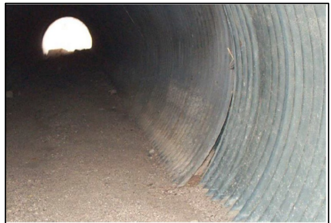
Joint Gap. Image Courtesy of Simpson, Gupertz & Hager
