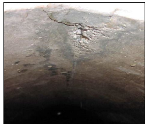
Spalling. Image Courtesy of Simpson, Gupertz & Hager
