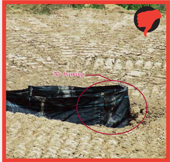
H. Drainage Inlet Sediment Control
