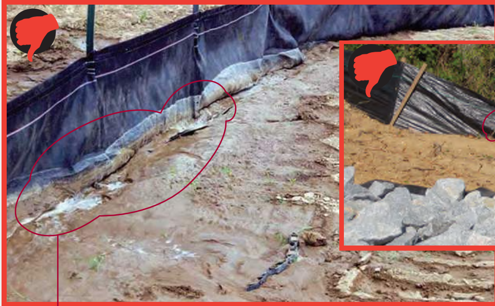
Anchor trench erosion
