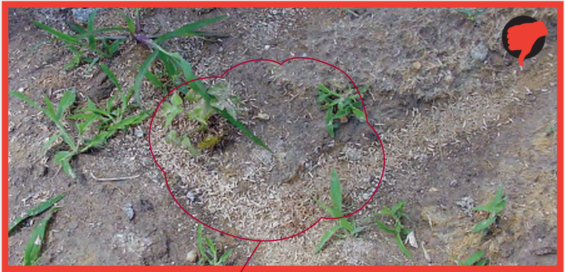
Poor seeding application
