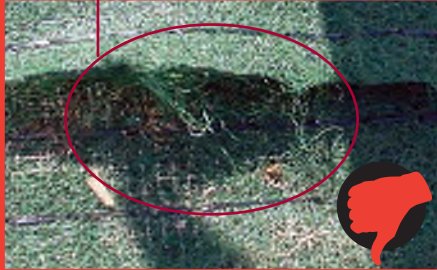
Improper stapling at overlap
