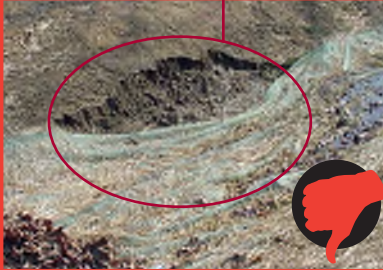
Failure due to no anchoring or stapling
