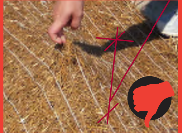
More than 6" indicates improper stapling. Staples not staggered
