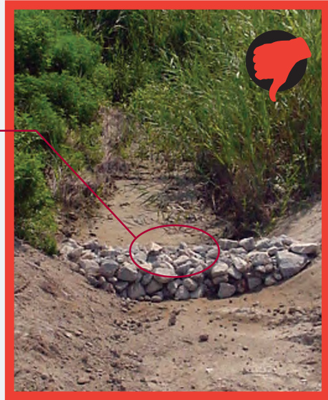
E. Stone Check Dam
