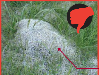
"Tenting" due to improper stapling
