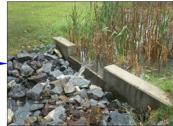
V-NOTCH WEIR / HAR01
