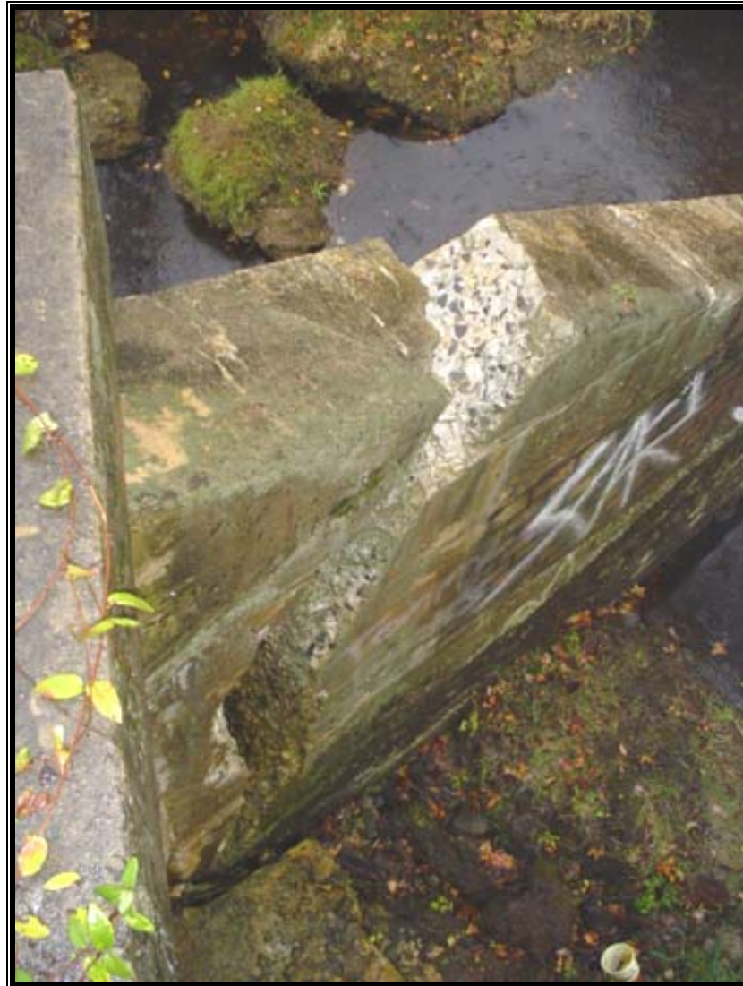
Fig. 7.3- Cracked south face – east wing wall
