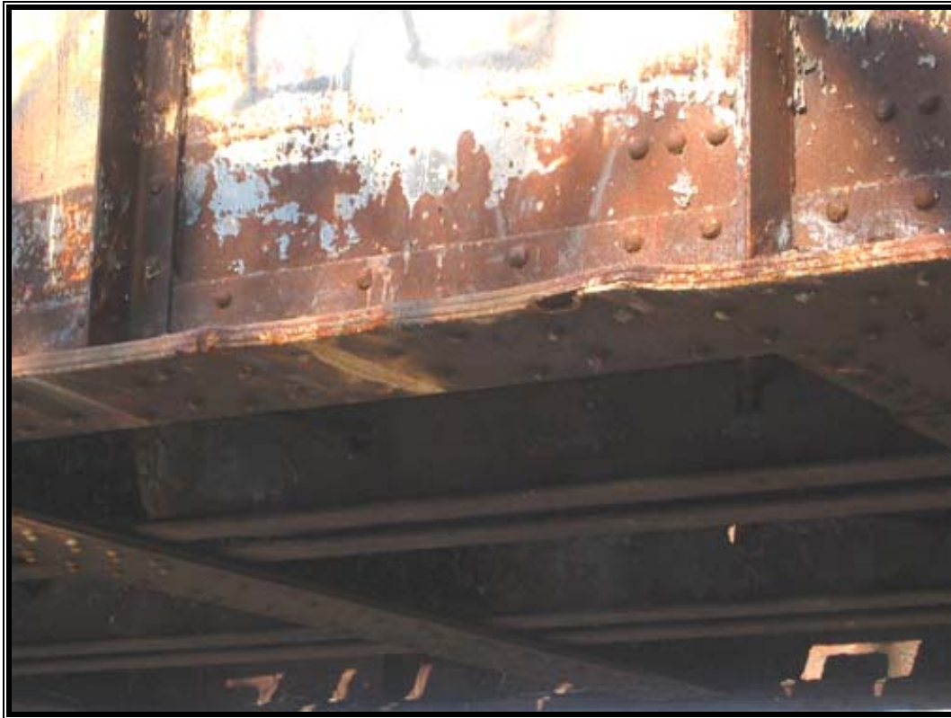
Fig. 9.2- Evidence of vehicular damage on south exterior girder
