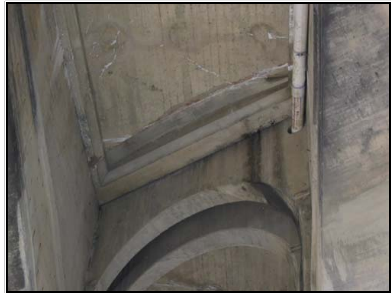
Fig. 4.4- Concrete repair with efflorescence
