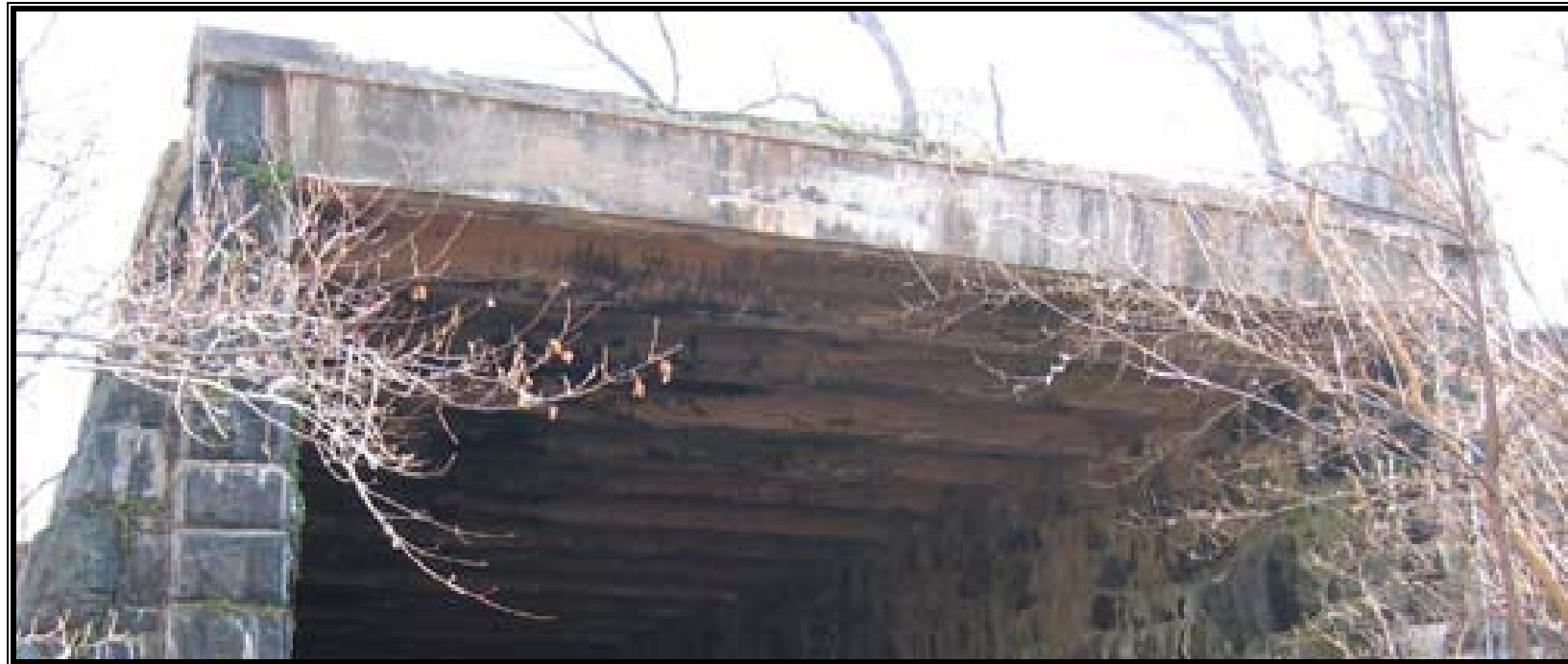
Fig. 8.2- Typical exterior beam cracking and efflorescence on west end
