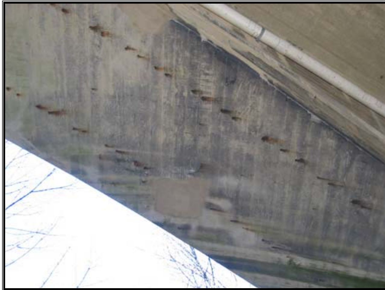
Fig. 4.3- Staining of rebar directly over area of proposed trail
