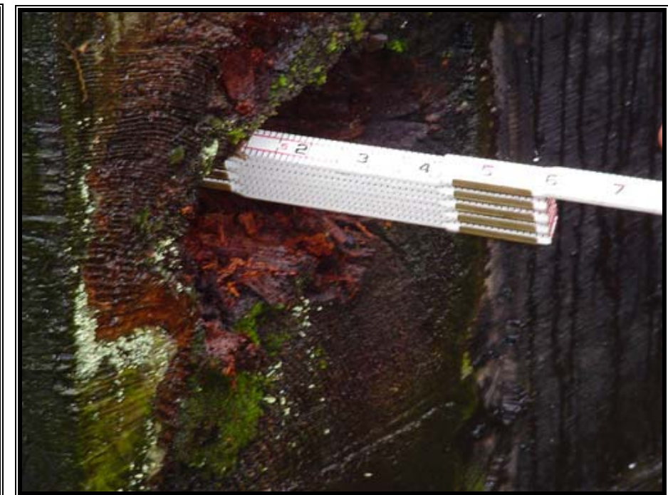
Fig. 5.6- Rot in wing wall 2'6" deep
