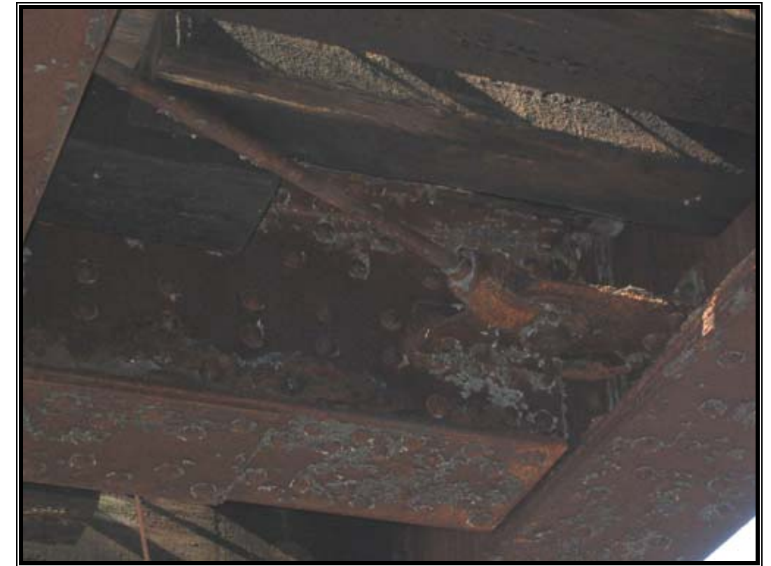
Fig. 9.3- Typical rust and paint flaking at strut and exterior beam
