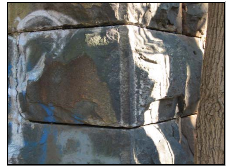
Fig. 9.7- Typical mortar joint damage
