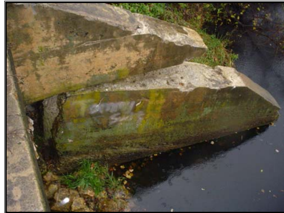
Fig. 7.4- Differential settlement at south face – east wing wall
