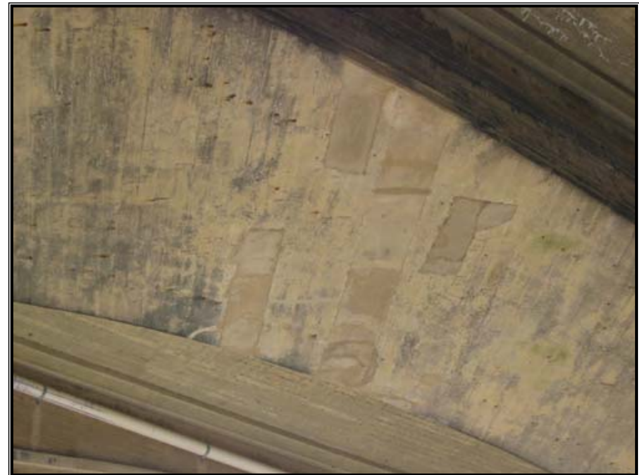
Fig. 4.2- Evidence of concrete repair directly over area of proposed trail
