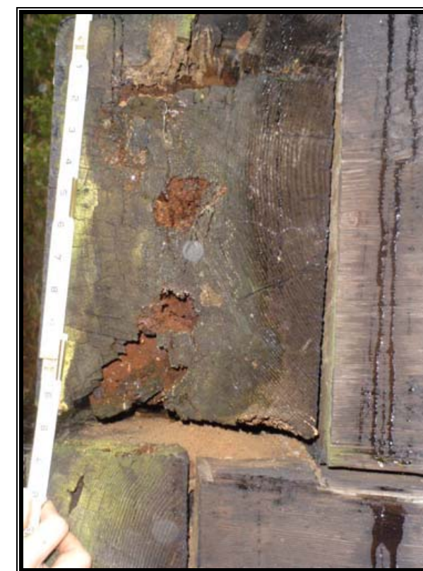
Fig. 6.3- Typical wing wall timber deterioration
