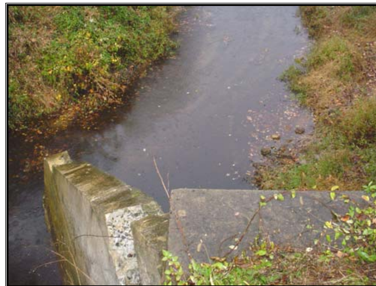
Fig. 7.2- North face –west wing wall directly in path of steam
