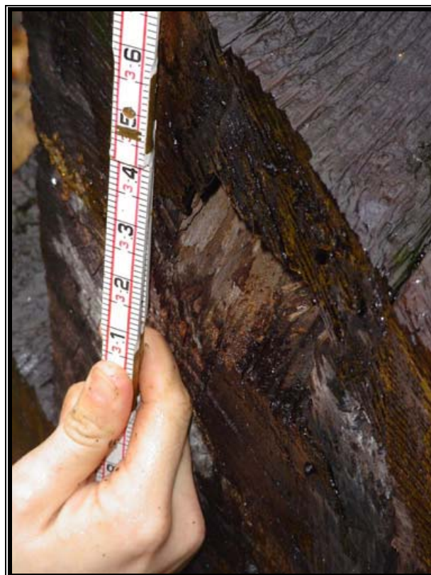
Fig. 5.7- Rot in wing wall 5 inches
