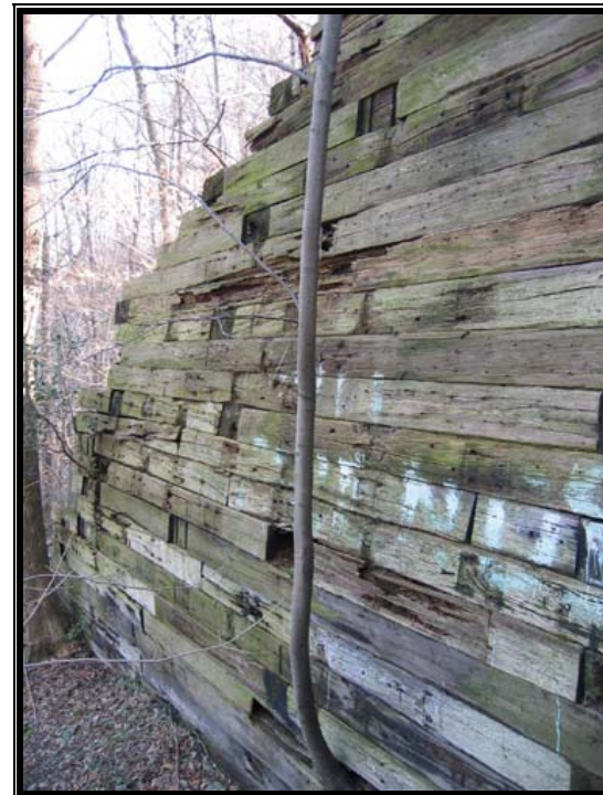
Fig. 9.9- Bowed north wing wall
