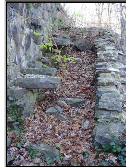
Fig. 8.3- Deteriorated stair case on north abutment
