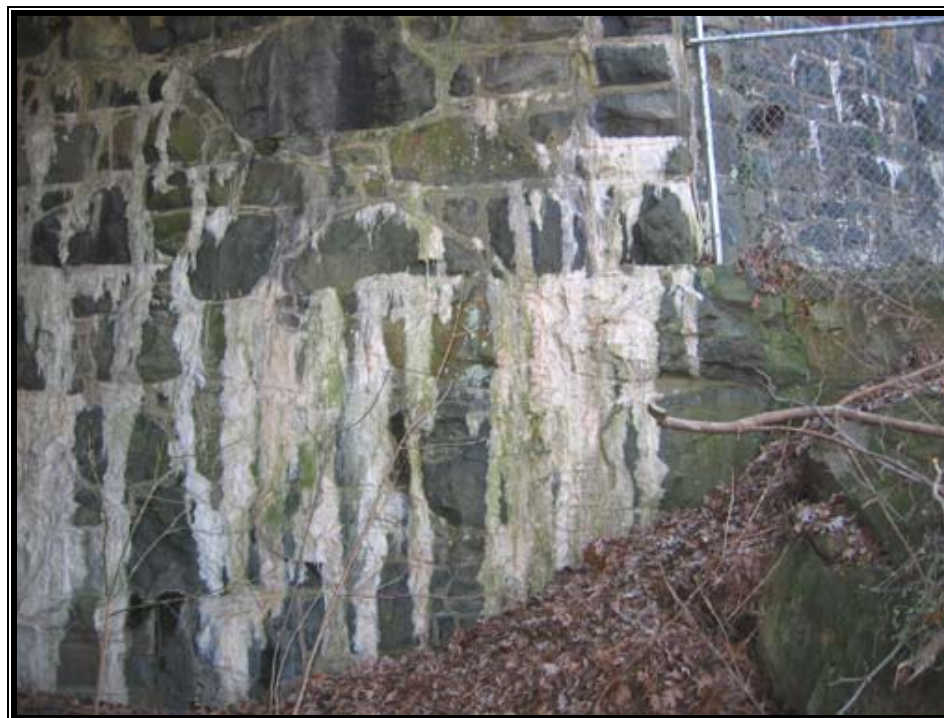
Fig. 8.5- Heavy efflorescence on south abutment – west end
