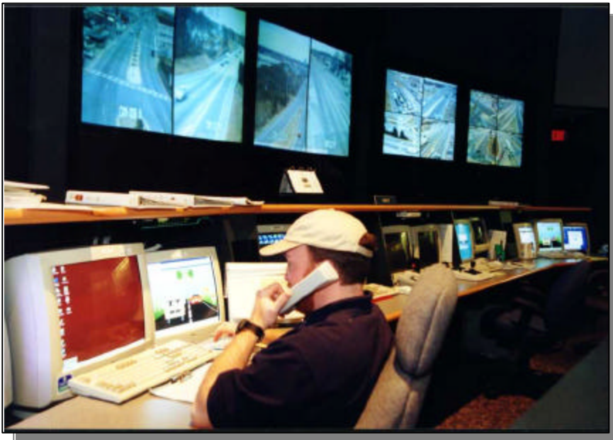
Transportation Management Center in Smyrna
