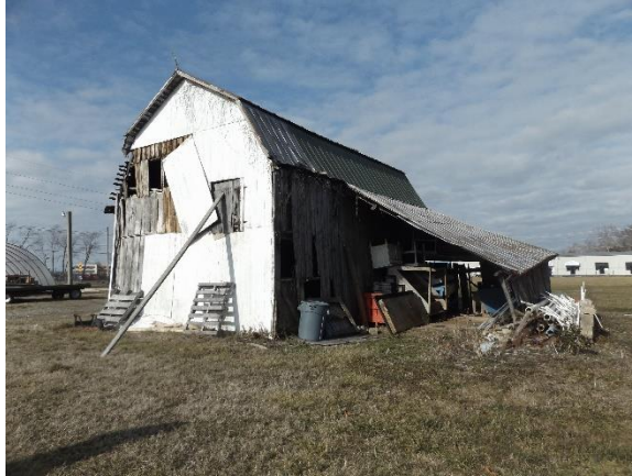
S00975 005 – View of the south and west (rear) elevation of the barn
