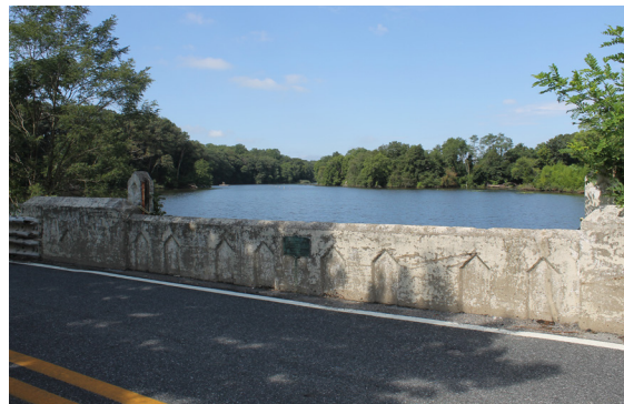
Detail of the west (upstream) parapet of Bridge 1-407, which features an incised diamond pattern and the original bridge plaque.
