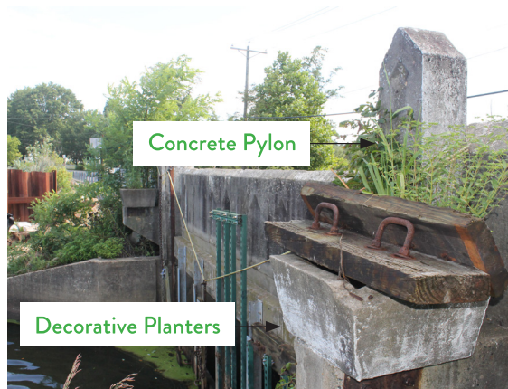
Detail of the concrete pylons and decorative planters featured on Bridge 1-407. Note the remnants of the metal stems and wood sluice gate boards, two of which are on top of a concrete planter.
