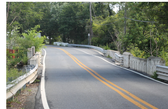
View of Bridges 1-407 (foreground) and 1-504 (background), which carry Silver Lake Road over the Silver Lake Dam and Spillway.
