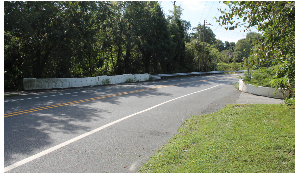
Bridge 1-407A carries Silver Lake Road over the Willow Grove Mill race.
