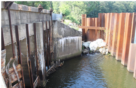
View of the temporary steel pilings installed to prevent Silver Lake from draining through the damaged sluice gates prior to repair.
