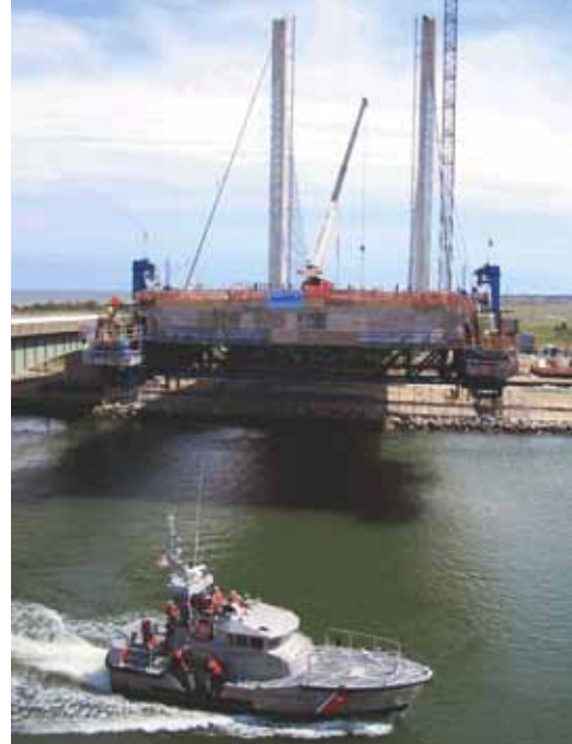
Boat traffic was uninterrupted as cantilever construction of the bridge extended out over the Indian River Inlet. Photo: AECOM.
