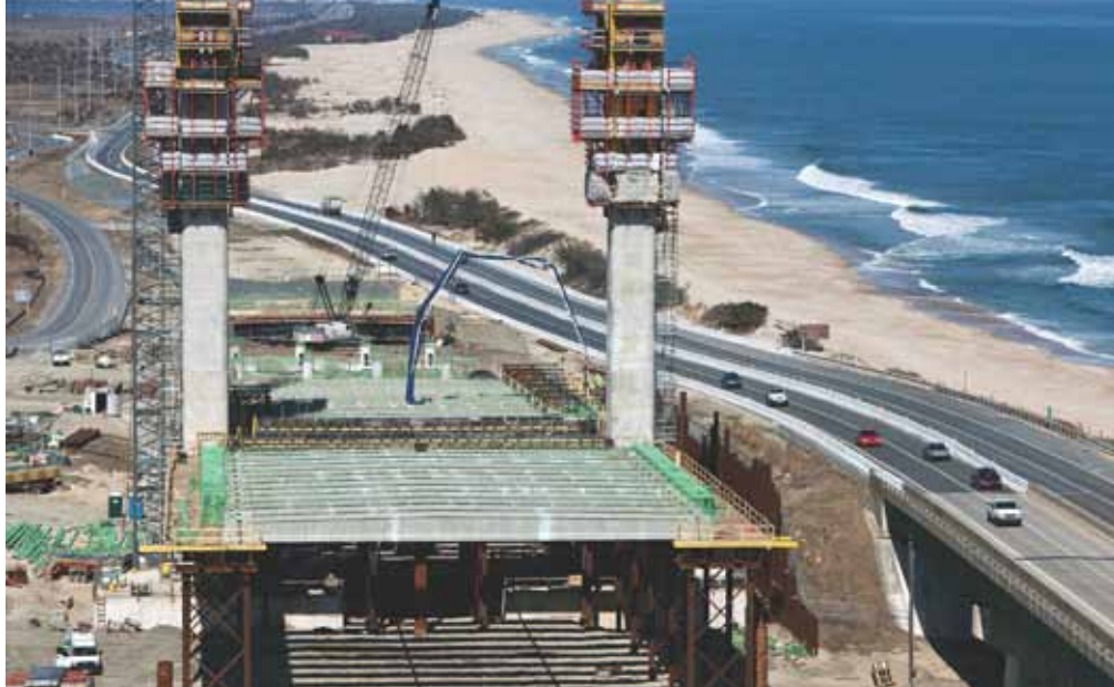
The use of precast concrete floor beams and cast-in-place construction on falsework for the portions of the bridge over land significantly sped construction because work could be completed simultaneously on several different fronts. Photo: AECOM.
