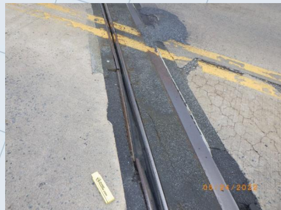
Spall in the barrier and missing steel plate
