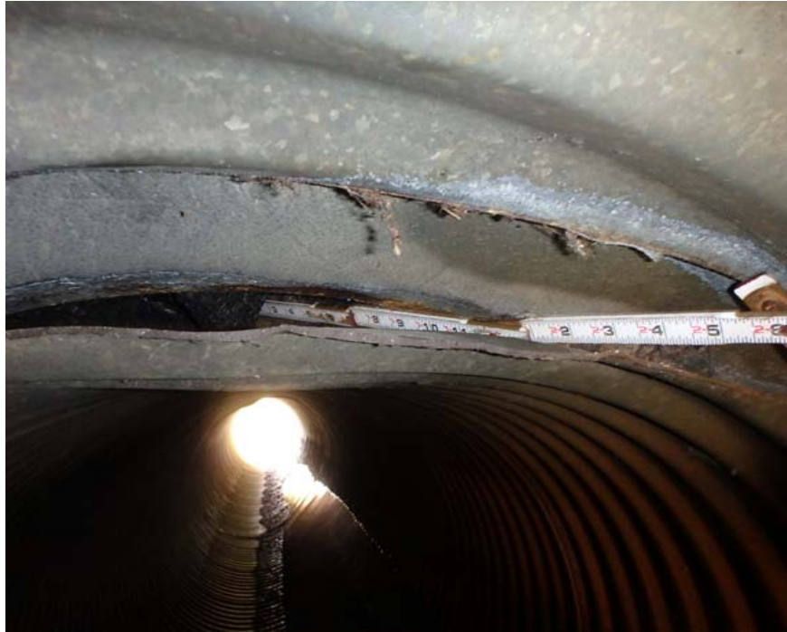
BR 2-066A Separation at 1st joint
